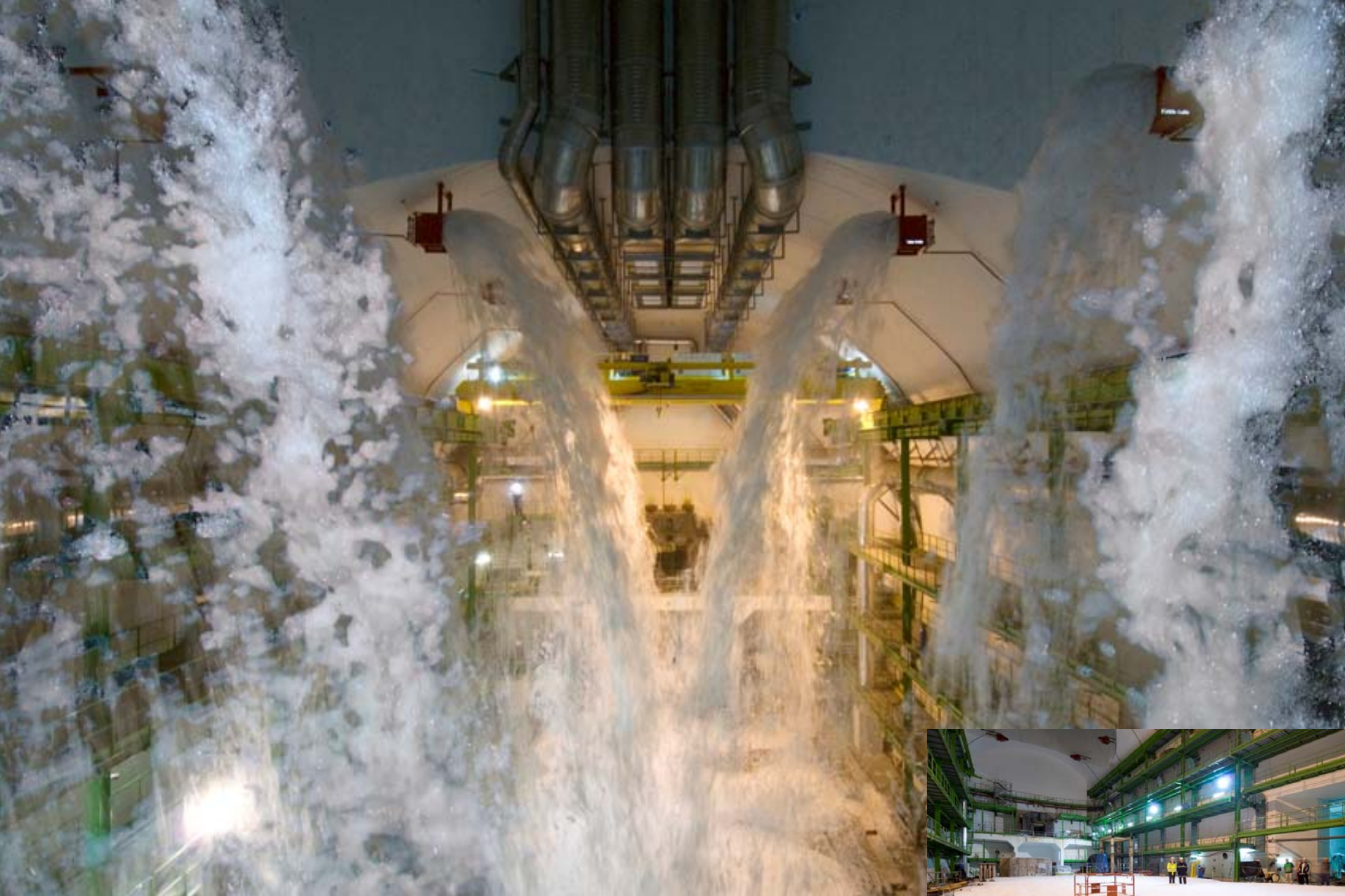
Test of the fire extinguishing system (12 May 2006)
