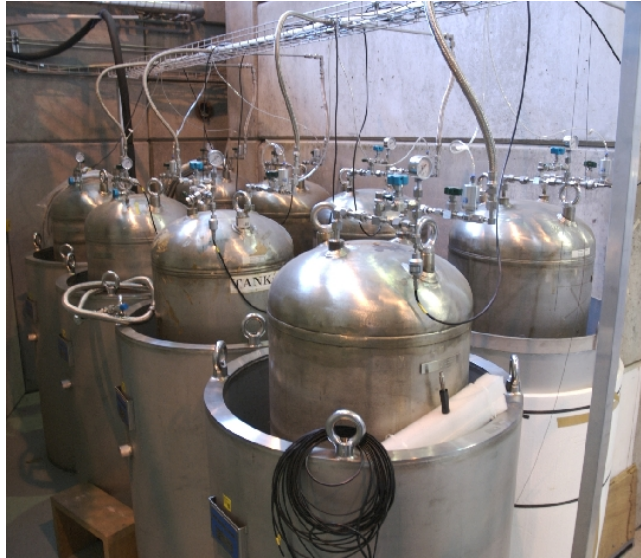
Figure 3.13: GXe storage tanks in the experimental area
